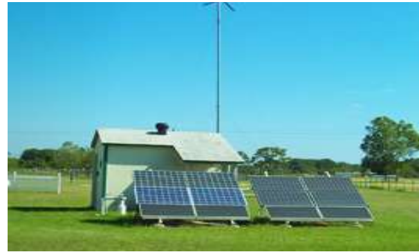
Ground-Mounted SED (Houston, Texas)
