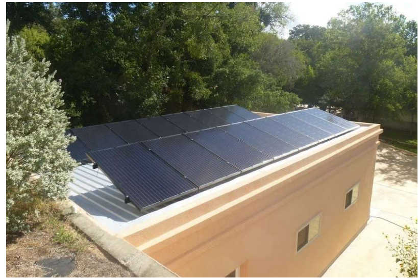
Tilted, Flat-Roof Mounted SED (Bastrop, Texas)
