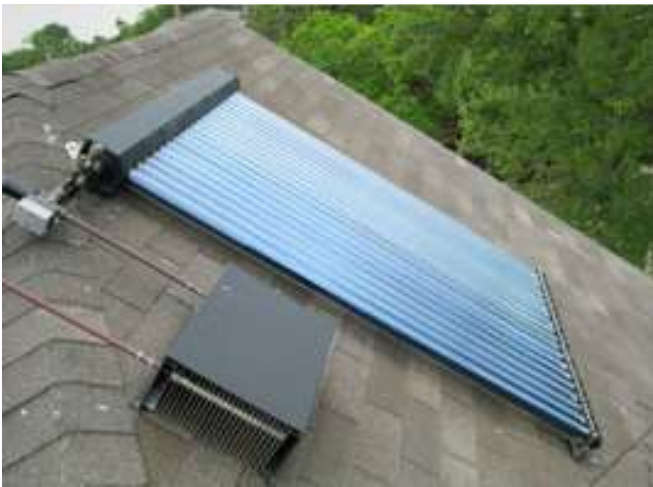
Solar Hot Water System (Houston, Texas)
