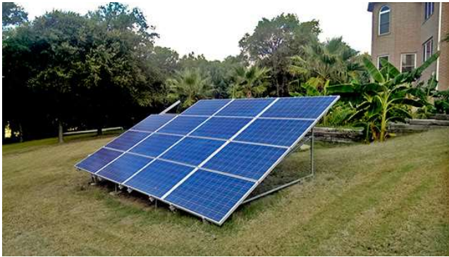
Ground-Mounted SED (Little Elm, Texas)
